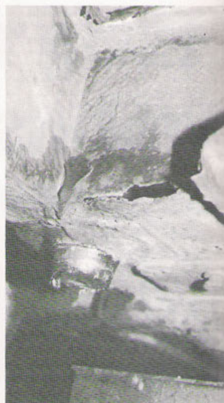
Rot is present on this 'E' type but luckily the radius arm mount is still in position. In severe cases, this whole section can just fall to the ground after a good burst of acceleration.
