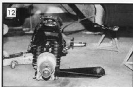
12 Here the rear end is positioned ready to be lifted in place.
