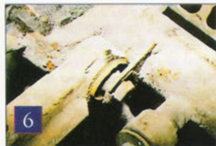
6 This rubber bush has become detached from the metal sleeve so that metal now turns on metal without the resilience of rubber.
