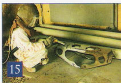
The replacement frame was meanwhile being shot-blasted to remove surface rust and grime. It was immediately coated in protective primer.
